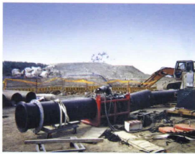
恆春海洋生態博物館新建工程 New construction project of Ocean ecological museum in Heng Tsun.
