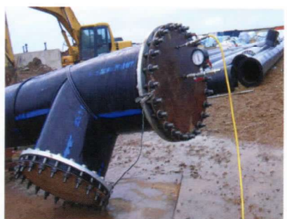
淡水BOT污水處理廠 Sewage Treatment Plant Project
