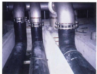
澎湖海水淡化廠 Plant for desalination process of sea water in Penghu.
