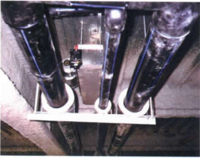
潮州鎮農會農民休閒教育中心空調工程 Air-conditioning project for Chao Chou Jeng Farmer's Association Leisure & Education Center.
