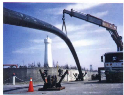
中油永安天然氣海放管工程 Chinese Petroleum Corp Yung An natural gas submarine piping project.
